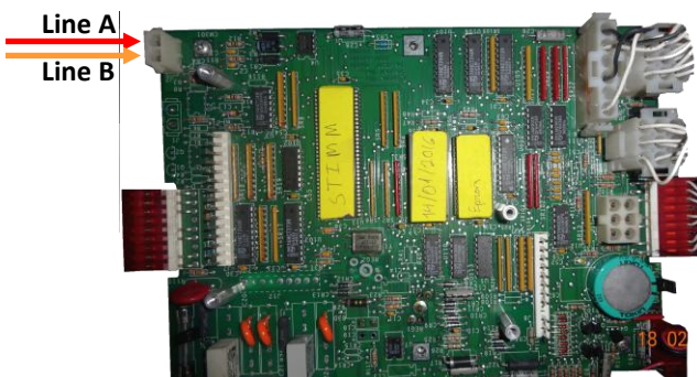
Wayne Dresser V387 dispenser board
